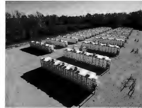
Dry Bridge Energy Center, 20 MW/80 MWh (Chesterfield, VA – owned by Dominion Energy)
